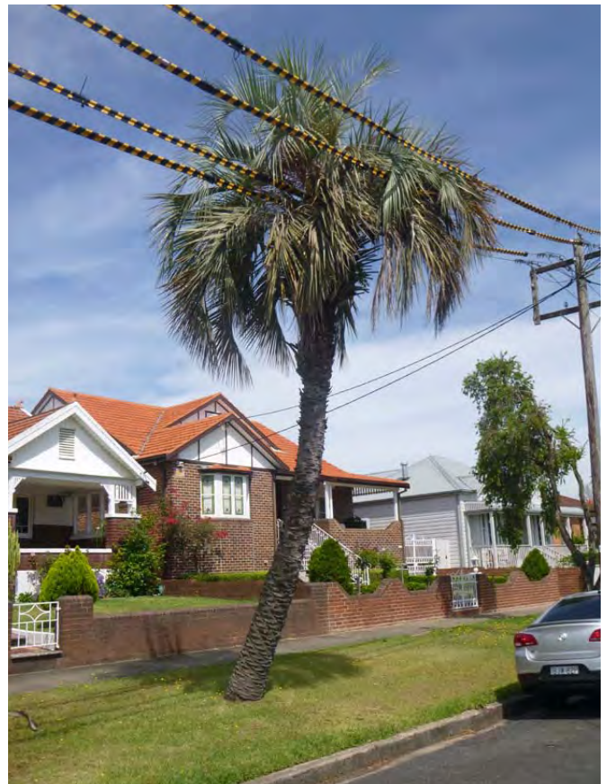
Figure 4.6 - The installation of ABC cabling above street trees may assist with retaining trees that may otherwise need to be heavily pruned or removed as a result of power line clearances. (Example - Martin Street, Dobroyd Point) (Photo - Arterra)
